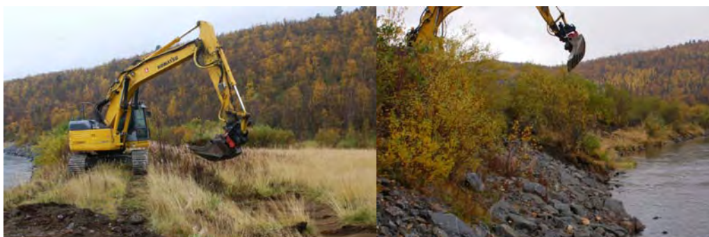
Figure 9.1 Excavator moving large and smaller vegetation mats with soil and growth substrate, completely covering the slope. Photo: Gunnar Kristiansen, NVE
