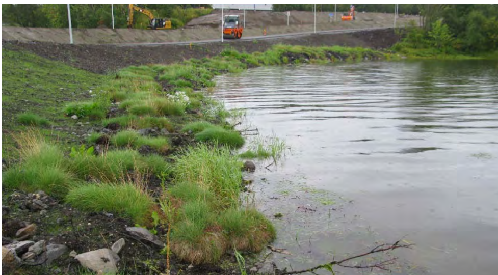
Figure 9.4 Moved turfs of sea shore vegetation in the transition between the outlet of Storelva and the tidal zone. The turfs was temporarily stored at the plant for approximately two years, the pictures show the site only weeks after they were placed out in 2013. Photo: Statens Vegvesen/v Elisabet Kongsbakk
