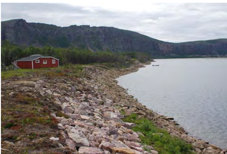
Figure 3.1.2 Erosion control construction in the outlet of the Tana River. Photo: Knut Aune Hoseth, NVE
