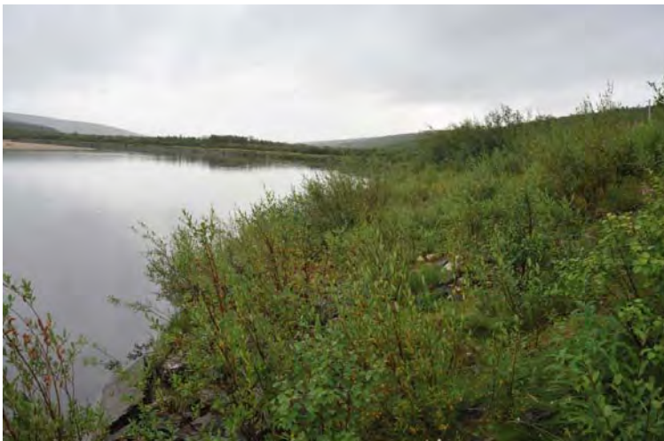
Figure 9.3 The erosion control construction at Jeabmelsnjarg before environmental measure. Moved soil and clusters of vegetation first year after the flood. Four years after measures where made show that a dense cover of vegetation has established. Photo: Gunnar Kristiansen, NVE
