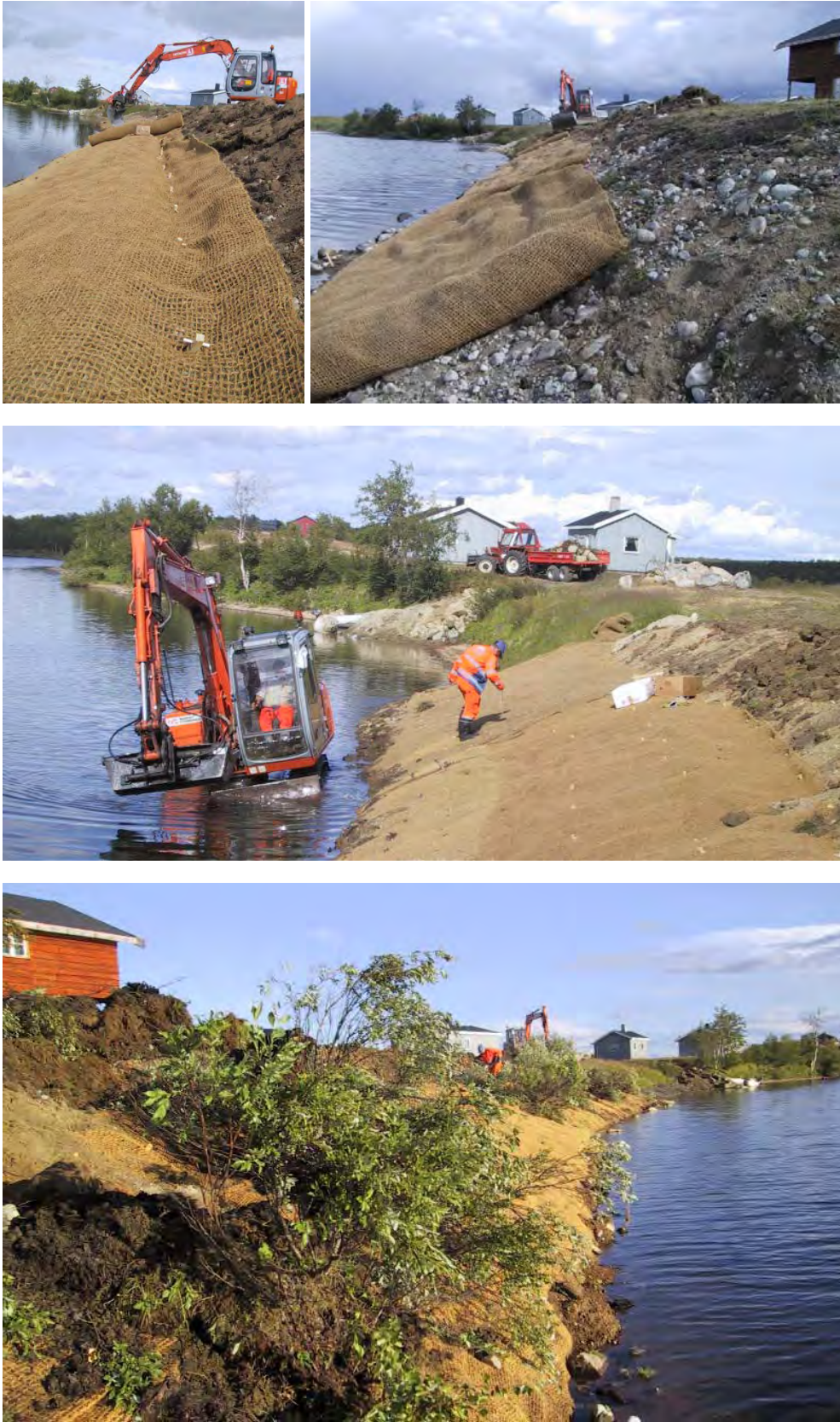
Figure 12.3 Erosion prone slope at Mollisjok along the tributary river Karasjohka, secured with geotextiles from further erosion of the slope. At this site soil and turfs of plants and bushes was moved over the slope immediately after applying the geotextile. Photo: Gunnar Pedersen, NVE
