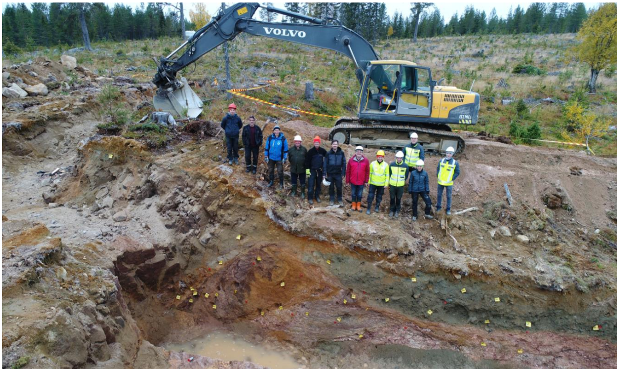
Figure 2. Ristonmäntikkö postglacial fault (location in Fig. 1). Photo by N. Nordbäck.
